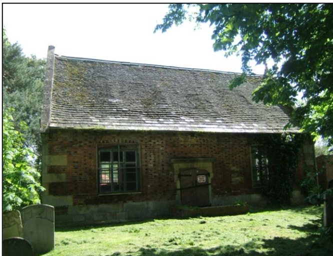
Fig.18 Bourne Grammar School is on the Council's internal Buildings at Risk Register.
