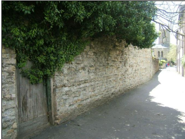
Fig. 16 Boundary walls of random rubble enclose the footway and create visual consistency along Church Walk.
