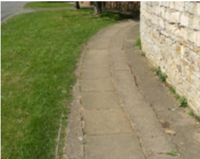
Fig.10 Historic Floorscape at Bottesford Road with attractive boundary wall to the right.
