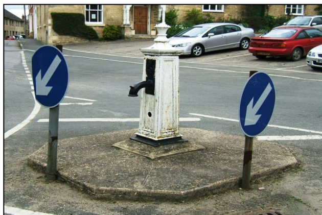
Fig. 8 inappropriately placed street signage has a negative impact on the listed waterpump.
